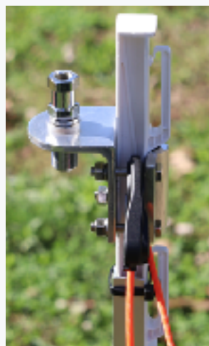
Notice the antenna anchor pole and easy on/off connection points for the antenna and coax connectors.
